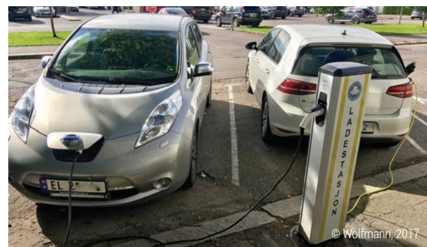
Figure 2.5: EV charging station in Storgata, Norway.
